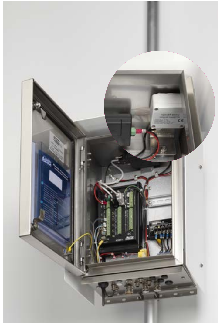
Example of installation in the housings for weather stations.
